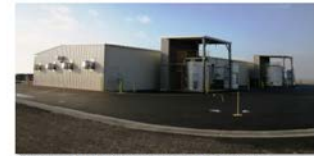
Operate 5 groundwater treatment facilities (pump and treat). Install two chemical barriers (apatite for strontium-90 and phosphate for uranium plumes)
